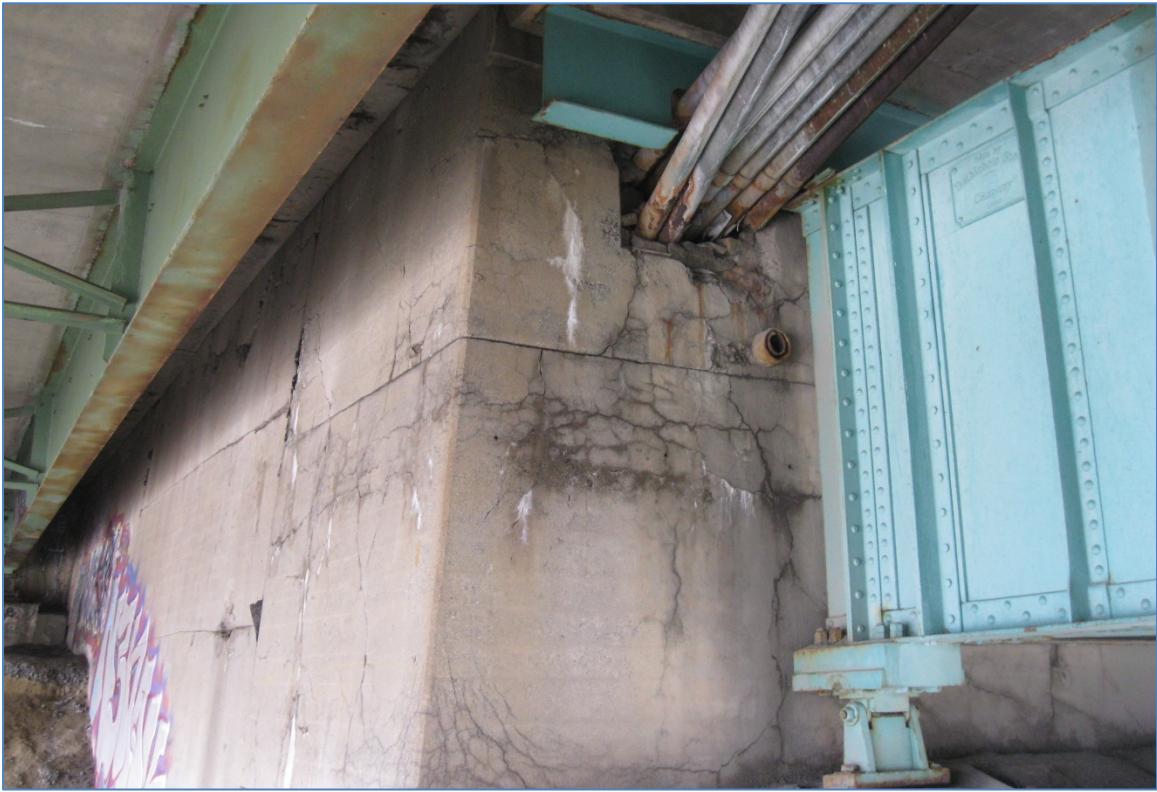
Figure 10 - East Abutment, Bridge Mounted Electric
